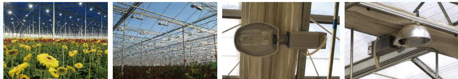
高压钠灯 High voltage sodium lamp
